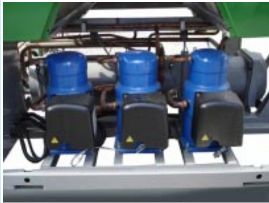
Multiple scroll, fully hermetic compressors.
