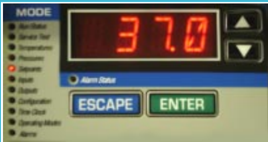
Scrolling marquee diagnostic display and control module.
