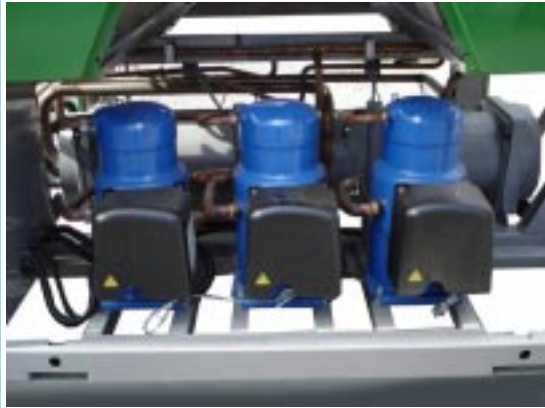
Multiple scroll, fully hermetic compressors.
